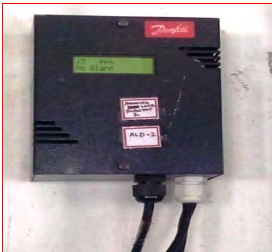
Ammonia leak detector that trigger alarm and put on ventilation fans
