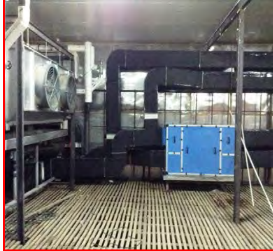
CO 2 / Air exchange system
