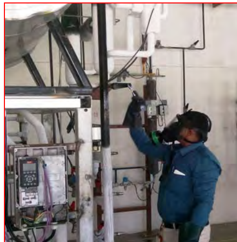
Worker fixing / attending ammonia leakage.
